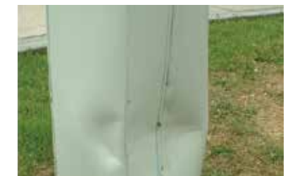
Photo 2.8 column visibly damaged
