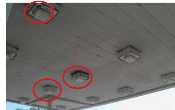
Photo 3.4 more than 2 light covers dirty
