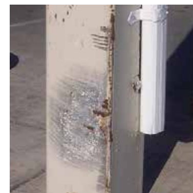
Photo 3.5 column dirty, rusty, damaged
