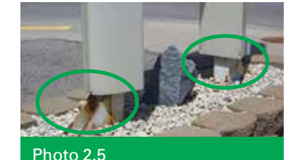
Photo 2.5 minor rust only at base of MID not visible from 15–20 feet away
