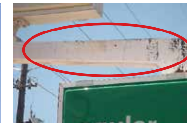
Photo 2.7 column rusted with paint chips
