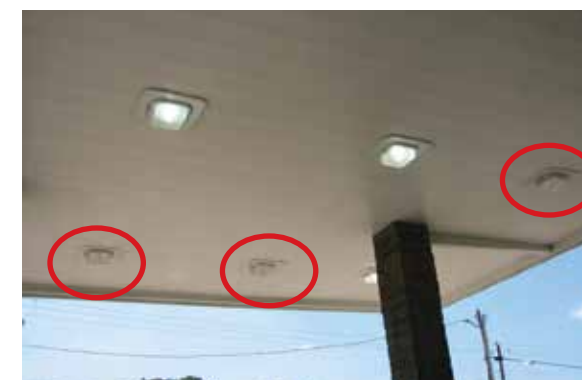
Photo 6.4 more than two canopy lights out
