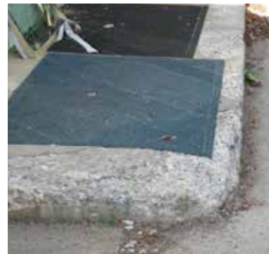
Photo 10.3 storefront curb damaged / crumbling concrete
