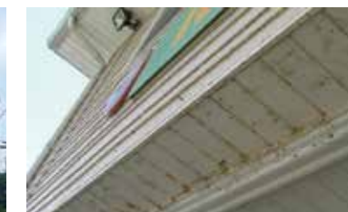
Photo 11.4 building exterior dirty
