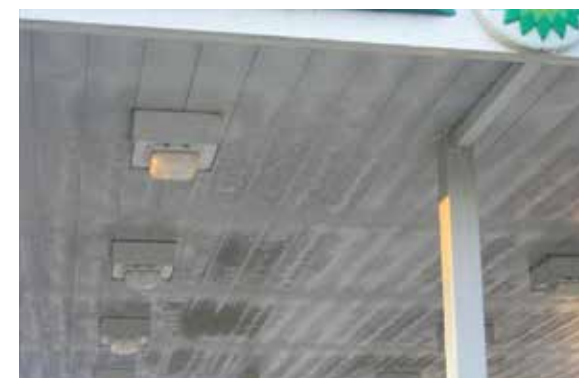
Photo 3.3 underside of deck with large areas of dirt
