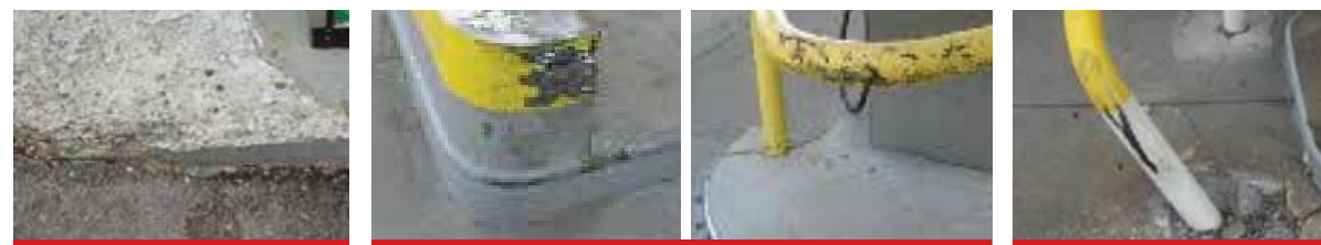
Photo 9.11 pump island damaged
