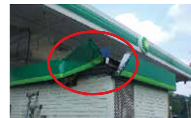
Photo 11.3 building exterior damaged
