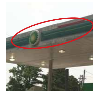
Photo 3.6 fascia peeling paint, dirty
