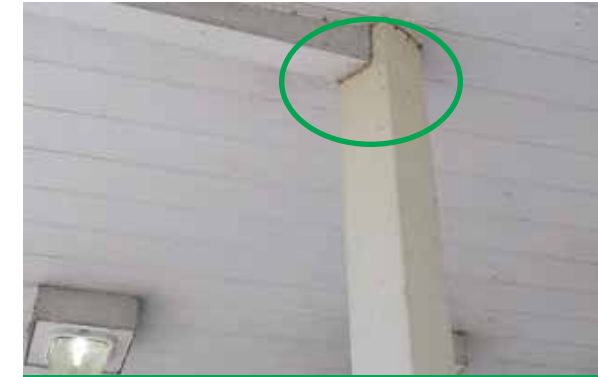
Photo 3.2 one column out of four with rust
