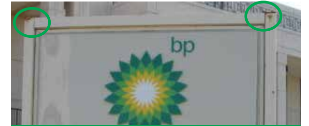
Photo 2.2 minor rust in two corners not visible from 15–20 feet away
